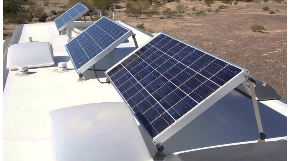
4x 250w PV Panels
